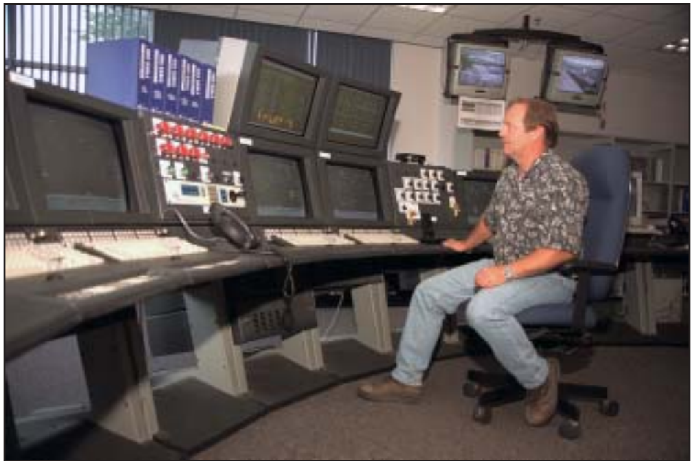
Dave Bernard, senior operator, monitors the whole plant from his seat in Aux Sable's high-tech control room.
